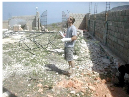
Joe with his new cast watching work on the tower. Background: New lines laid out waiting for prep prior to installing.
