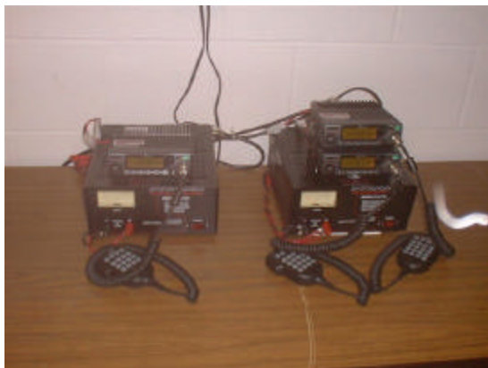
A view of the OMMRS Radios that were installed at Immanuel Hospital.
