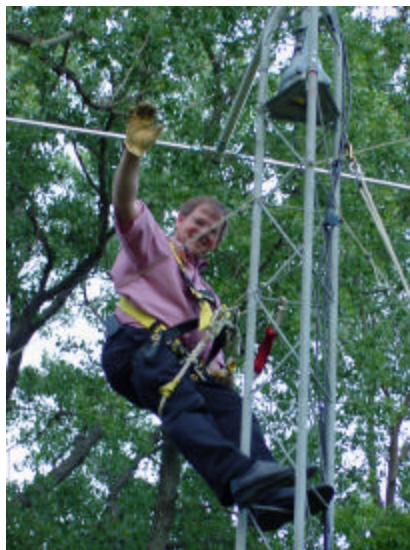
Rick, AAØH, was this years volunteer tower climber and put up the lights for night time illumination.
